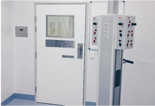
Lead Equivalent Glass Viewing Panel in lead lined door.
