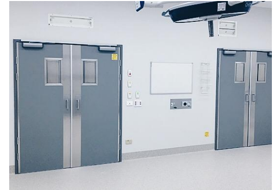
Lead Lined Impactboard wall with Lead Lined Doors.
